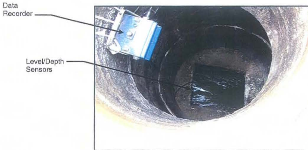
Figure 3-5 Typical Flow Monitor Equipment Installation
